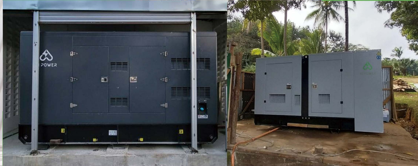
Industrial area in Philippine 300KVA Cummins with ATS Silent Type
