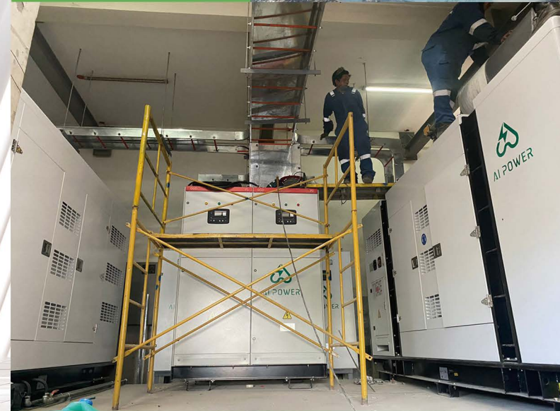
Industrial area 500KW*2 units with Synchronous system Perkins Silent Type
